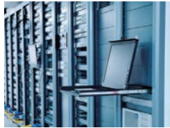
Control Room/ Data Center
