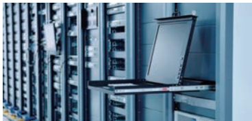
Control Room/ Data Center
